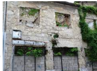
War damaged buildings in Mostar
